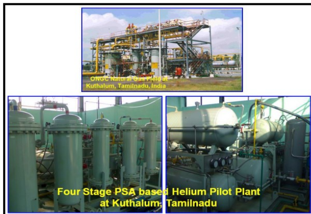
Figure 9: Four-stage PSA Helium Plant (proto type) installed at ONGC’s gas field (Karaikal Asset) at Kuthalam, Tamilnadu.
