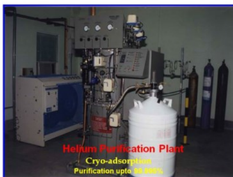
Figure 8: Helium Purification Plant installed at SINP/VECC Campus, Kolkata.
