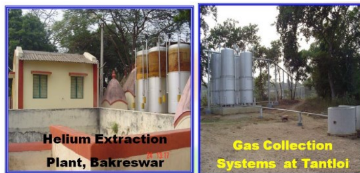
Figure 7: Photographs of helium plants installed at Bakreswar and Tantloi.
