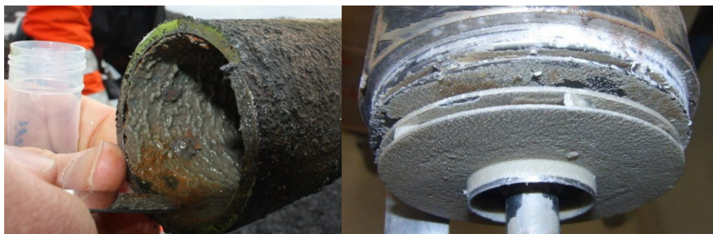
Figure 11: Calcite precipitation observed on monitoring equipment situated down hole in monitoring well HN-04 at the CarbFix 1 injection site. Left figure shows how the pipe going from the downhole pump and up to the surface is covered in greenish colored precipitation which was measured to be calcite ( \text{CaCO}_3 ). The greenish color of the precipitate is believed to stem from remnants from Na-Fluorescein tracer test carried out at the injection site (see Figure 2b). The right figure shows calcite precipitation inside the downhole pump. (Photos: Sandra Ó Snaebjörnsdóttir and Ingvi Gunnarsson).
