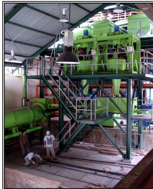
Figure 2: Palm sugar processing unit using 4 tonnes/hour brine from Lahendong geothermal power plant.
