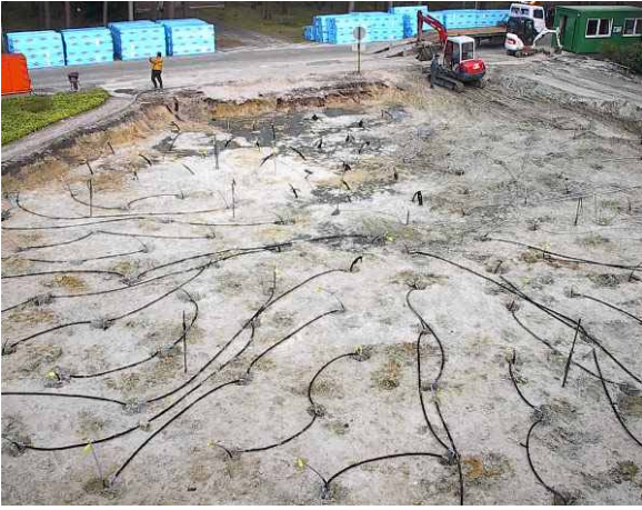
Figure 9: Storage field, hydraulic connection vertical heat exchangers (3 in series)
