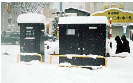
Figure 14: Control box (left) and heat pump (right) of the West Unit.
