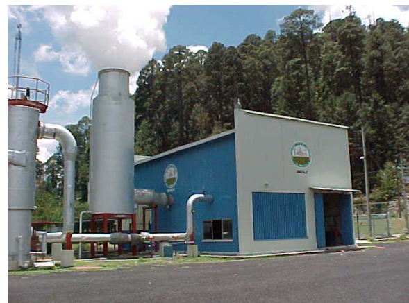
Figure 6: Backpressure unit of 5 MW
