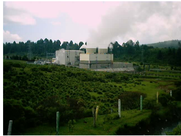
Figure 9: Condensing unit of 25 MW
