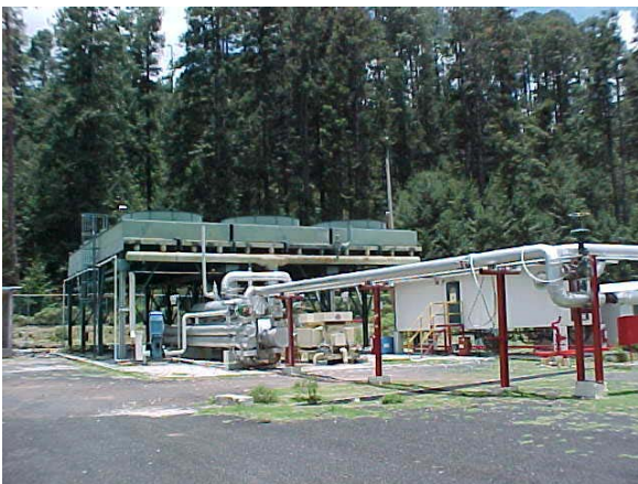
Figure 8: Binary cycle unit of 1.5 MW
