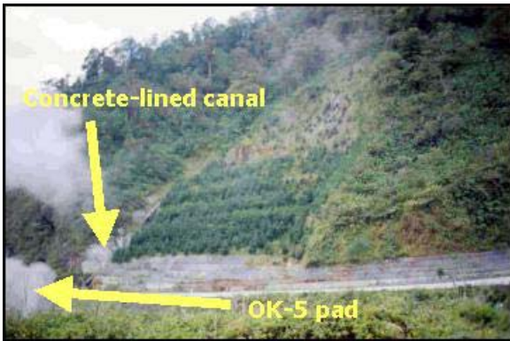
Figure 8: This is the massive concrete retaining wall constructed near the OK-5 pad periphery in SNGPF where a former landslide obliterated the OK-5 geothermal well pad. Note the bare slopes above the slide planted with trees and the concrete-lined canals beside the wall.
