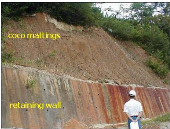
Figure 10: The view shows an example of vegetative stabilization in combination with rigid structural barriers being implemented in SNGPF near NJ-A pad. Here, coco mattings were installed to promote revegetation of the bare slopes above the retaining wall.
