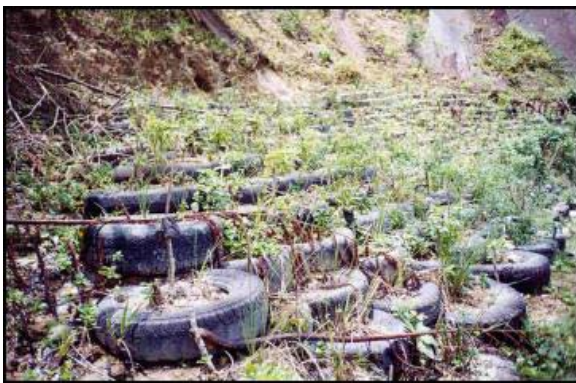
Figure 9: Old tires were overlain here in this photo near NJ-A pad periphery in SNGPF to reinforce the toe of the slope where a former landslide had occurred.
