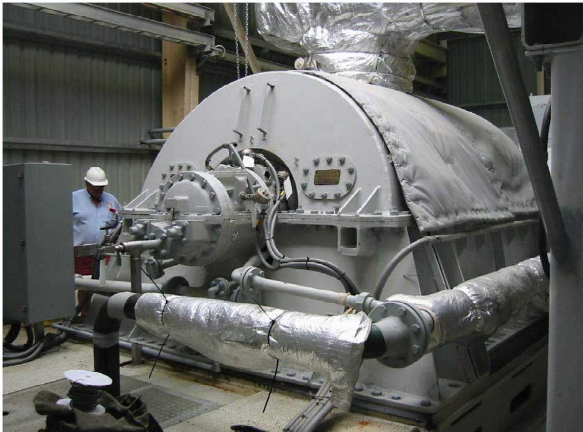
Figure 2. 6 MW Backpressure Turbine Unit
