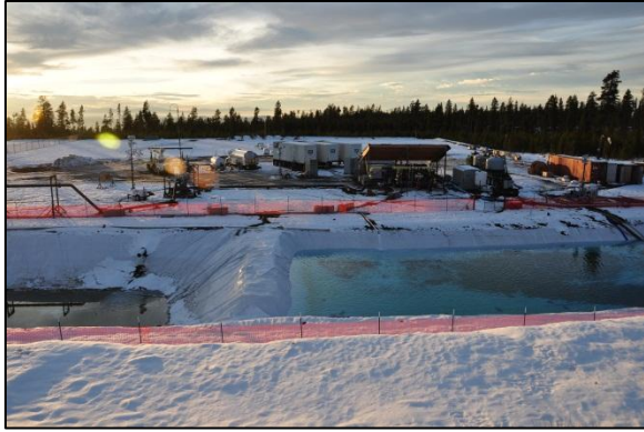
Figure 2: Newberry stimulation site photo. Showing from right to left, booster pump system, stimulation pump, high-pressure piping, TZIM injection system, wellhead assembly, and flowtesting set-up
