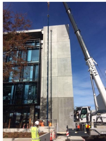
Figure 3. ECan submersible extraction pump suspended from crane.
