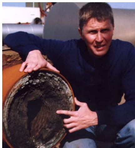
Figure 8: Calcite scaling in surface pipes
