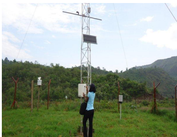
Plate 1: Automatic weather station at Menengai project site
