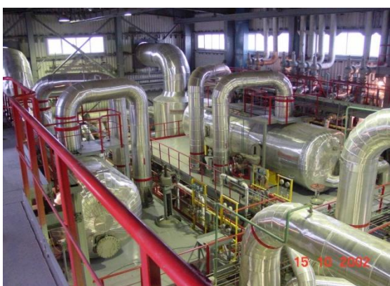
Figure 8: Separator's building of Mutnovskaya GeoPP.
