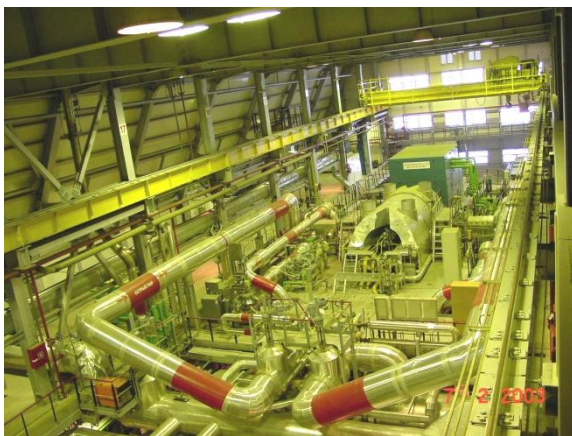
Figure 7: Main building of Mutnovskaya GeoPP.
