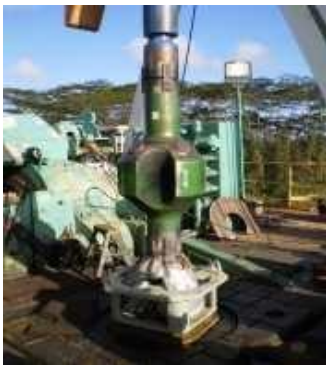
Figure 43: Specific stabilizer designed by Geothermal Resource Group
