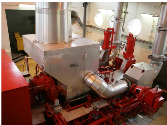
Figure 10: Fuji 6 MW backpressure turbine (Yamaguchi, 2010)
