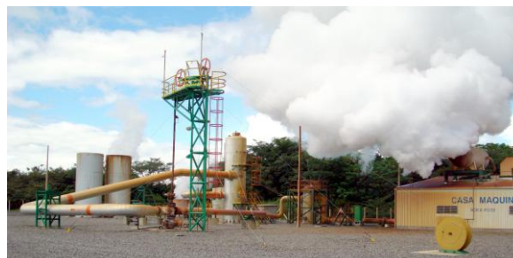
Figure 11: Miravalles PGM-29 wellhead unit and separator station (Moya and DiPippo, 2010)
