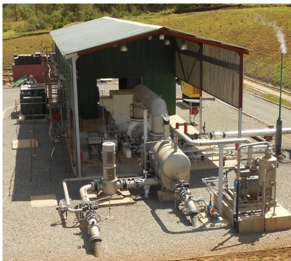
Figure 12: Eburru wellhead power plant with condensing turbine (Mendive and Green, 2012)
