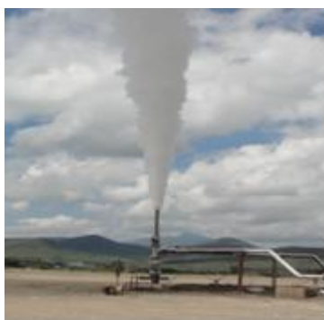
Figure 29: Photo showing OW-38B discharging into the atmosphere. The well has a discharge capacity of 18MW
