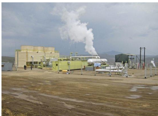
Figure 5: Photo of the 2.5MW Olkaria wellhead generator
