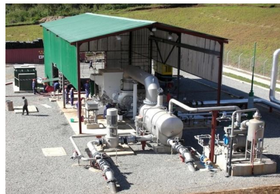
Figure 4: Photo of the recently commissioned Eburru wellhead power plant
