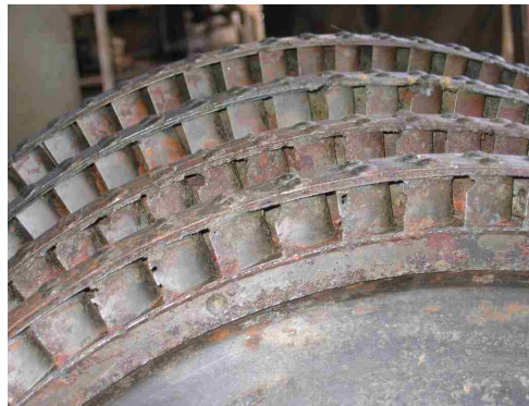
Figure 1: Corrosion of the turbine blades
