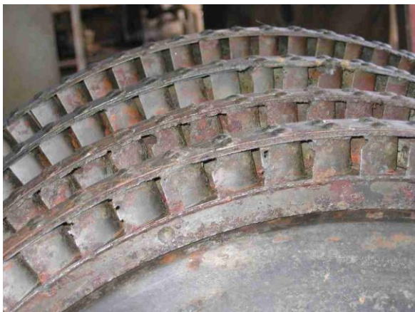
Figure 2 Corrosion of the turbine blades
