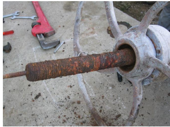
Figure 6 Corroded stem of a wellhead valve
