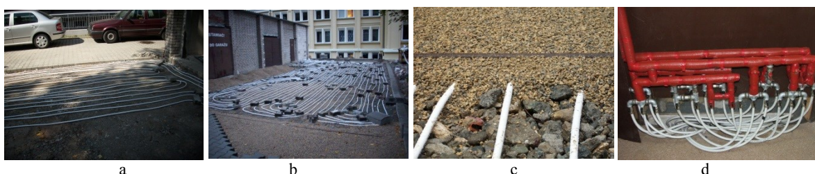
Figure 9: Tube loops in sand under the bricks, a,b,c - views at various stages of work, d - distribution installation of heating loops in the parking.
