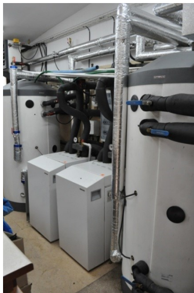
Figure 5: Two Stiebel Eltron heat pumps, a – heat pumps with switchboard and electrical energy counter, b – heat pumps with heat receivers on the left, and cold receivers on the right.
