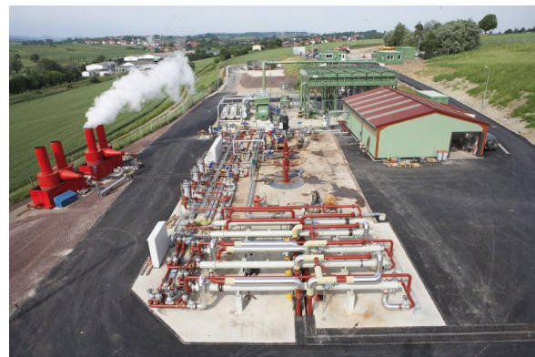
Figure 7: The Soultz geothermal power plant: in the back, the ORC power unit; in the middle, the 3 geothermal wells; in the front, the cooled geothermal loop.
