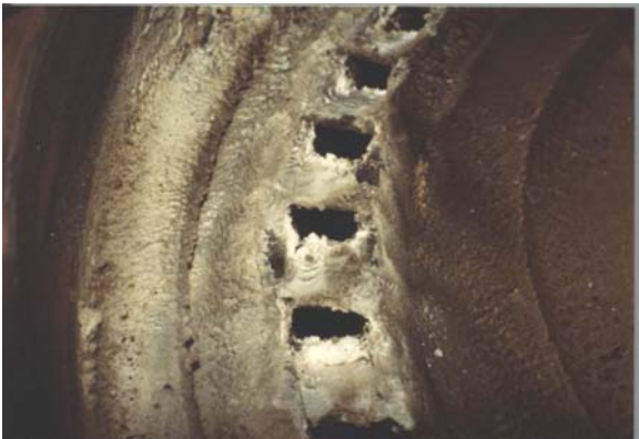
Figure 11: Steam turbine inlet nozzles with intensive scaling.
