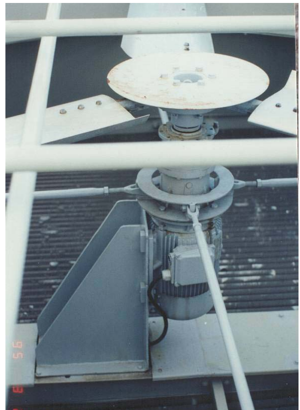
Figure 13: ORC cooling fan with gear motor.
