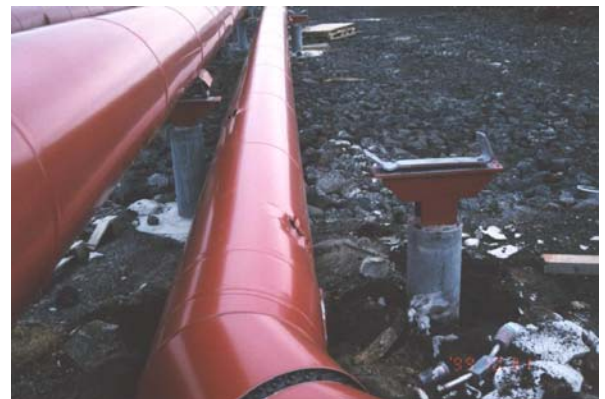
Figure 7: Slug flow knocked the pipe off its supports.
