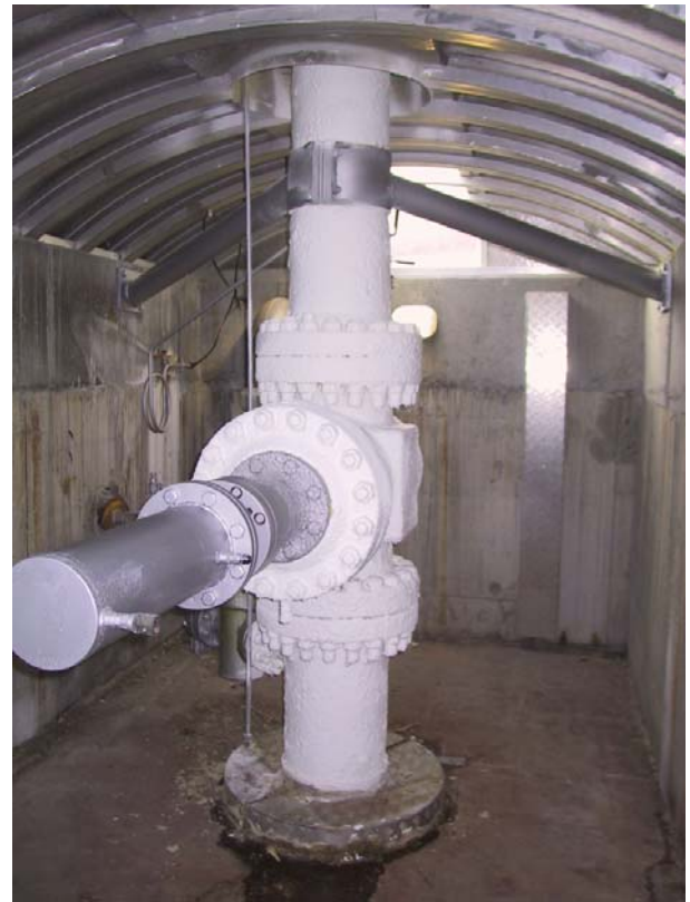
Figure 6: Wellhead master valve with hydraulic jack and spray on insulation.
