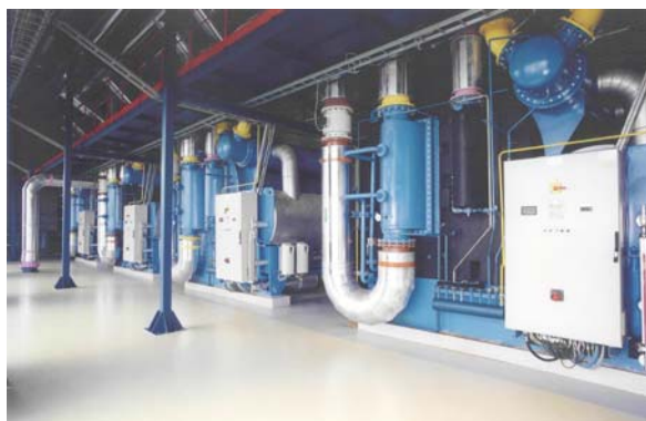
Figure 10: Absorption heat pump at KGDP.
